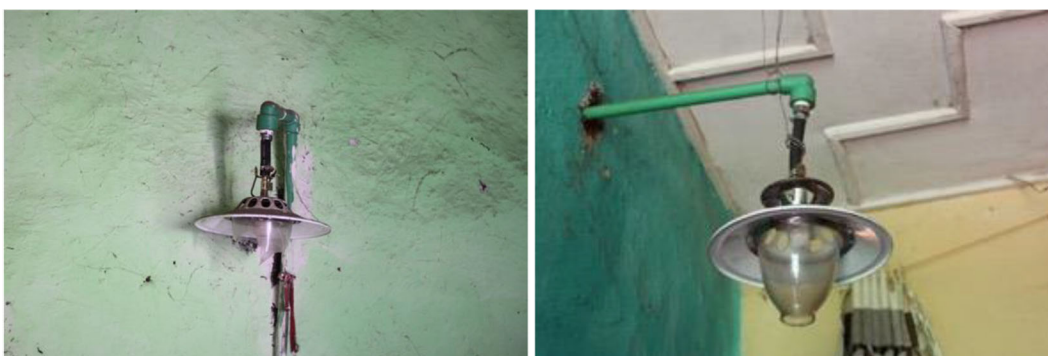
Picture 6 A broken biogas lamp compared with a functioning biogas lamp. Source: Own
